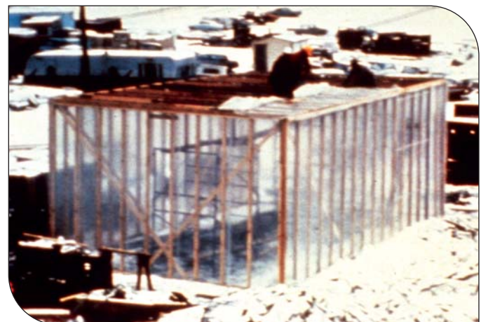
Figure 4. A temporary shelter protects the mortar preparation area from rain and snow. (IMG24817)
