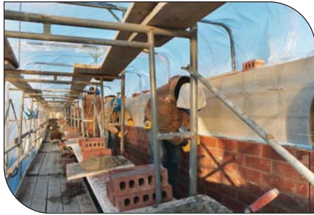
Figure 5. Enclosure and heating of a work area protects materials, workers, and installed masonry from severe weather. (IMG12508)
